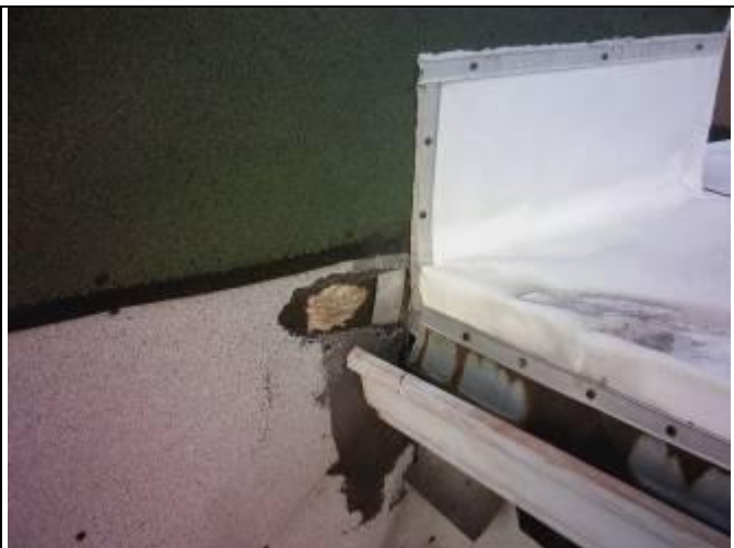
29. Damaged parapet wall covering and flashing at Building 115 north elevation
