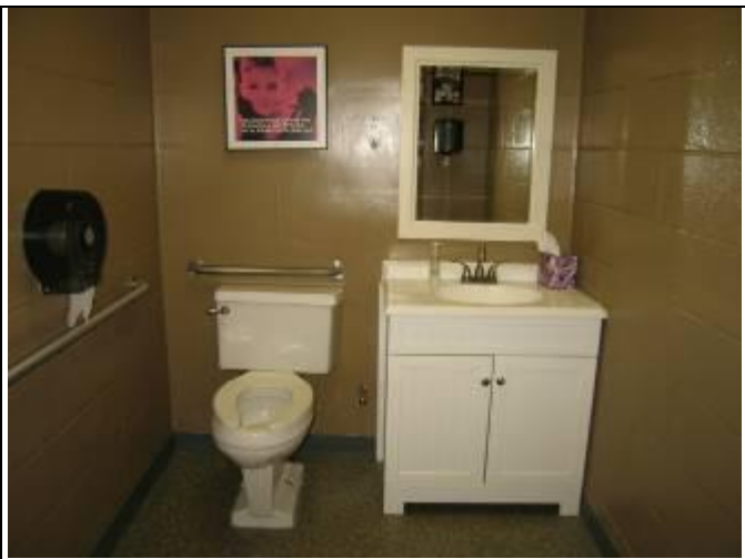
75. ADA accessibility view 5: Building 115 public access unit A ladies toilet vanity prevents access by wheelchair occupant – lavatory must have space beneath to allow leg room – pipes must have insulation to prevent leg abrasion – door widths and turnaround space appears satisfactory
