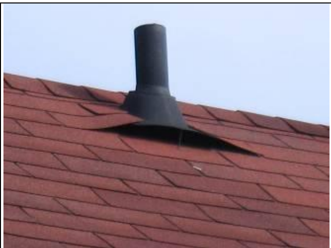
35. Building 113 waste vent boot requiring re-installation (has nail pop)
