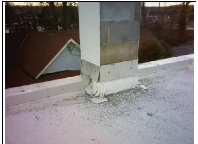
28. Damaged flashing at TPO membrane/block chimney
