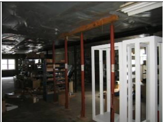
57. Structural view 5: Screw-jacks with drop-girders provide additional roof deck bracing in two location in the 115 Building unit A second floor
