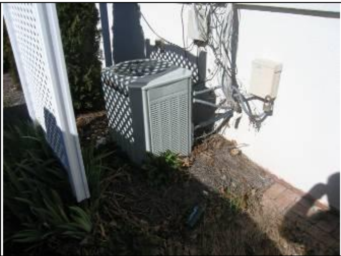
39. Typical Trane heat pump unit with Air Handler in crawlspace – date of manufacture 1989 (1 of 4 units)
