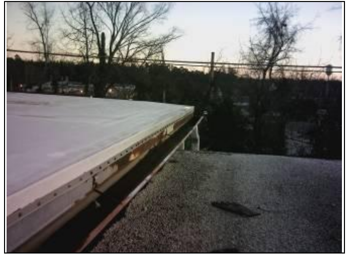
32. Damaged gutter at Building 115 TPO – BUR transition – area of active leakage directly below
