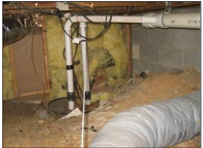
52. Sump-pump located in Building 115 crawlspace adjacent to unit D toilet area –unknown purpose
