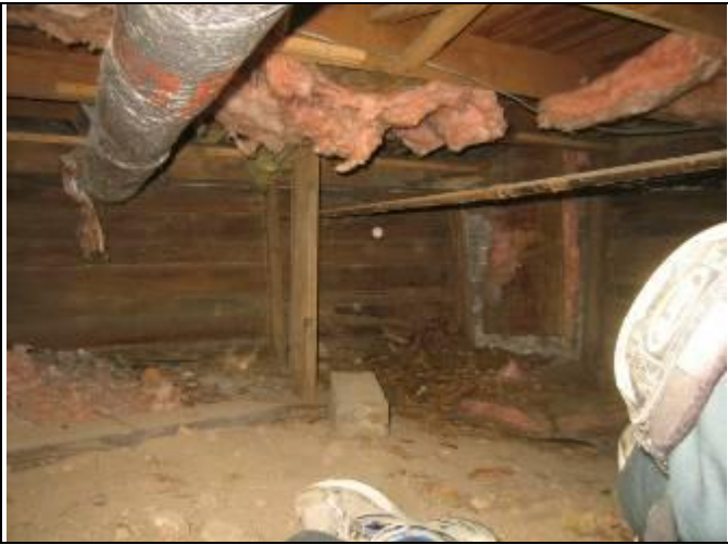
67. Structural view 14: Building 113 Crawl space: Wooden braces from soil to floor framing are a direct invitation to termites into the floor framing
