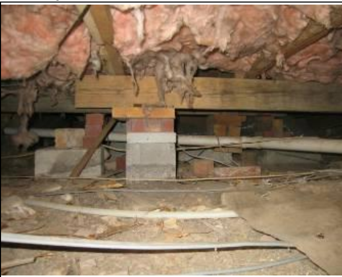
69. Structural view 16: Building 113: Stacks of brick, block, rocks and wood supporting numerous drop-girders providing bracing for floor framing
