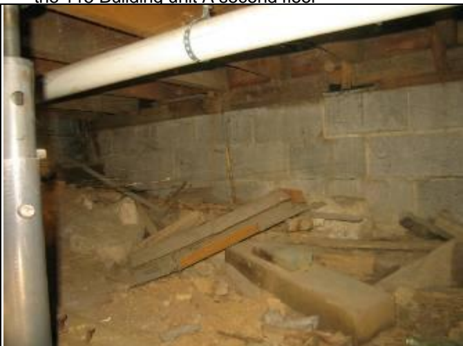
59. Structural view 7: Termite activity continuing down south crawlspace wall in Building 115 – Debris
