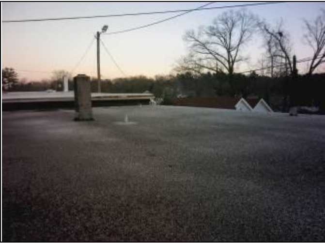
25. Gravel covered asphalt membrane view southeast – damaged gutter at upper left along TPO/BUR
