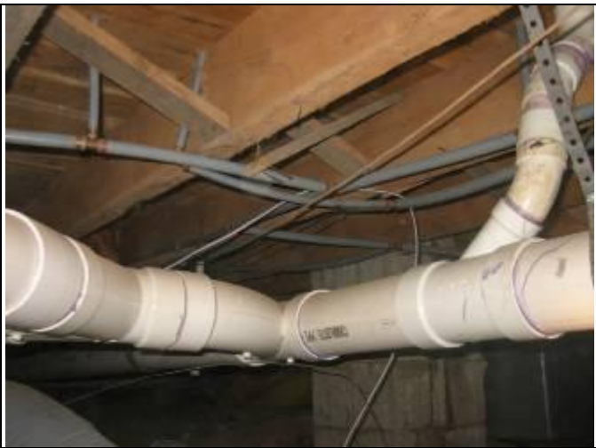
51. Polybutylene distribution and PVC waste piping utilized in Building 115 crawlspace
