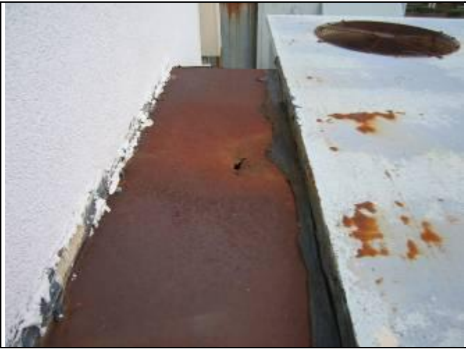
37. Damaged shroud at active Trane "gas-pack" HVAC unit at Building 115
