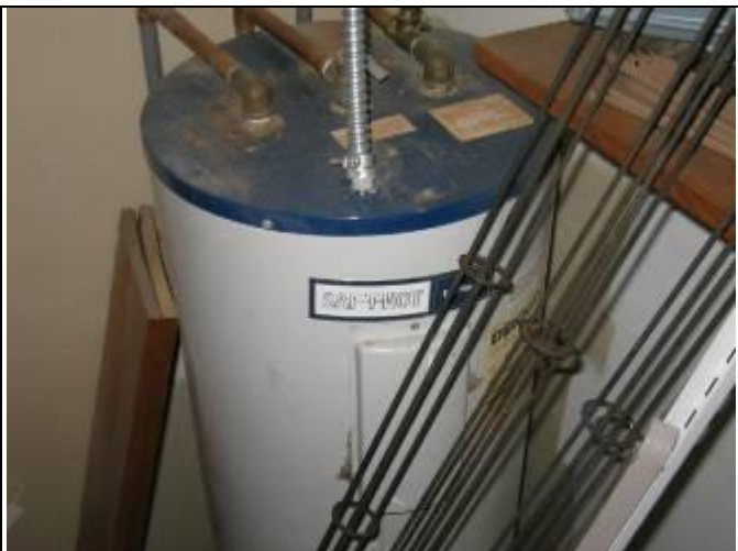
47. Electrically fired hot water heater in unit B – Building 115
