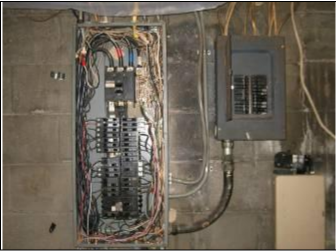
43. Distribution/service panel interior examination – Unit A Building 115 second floor
