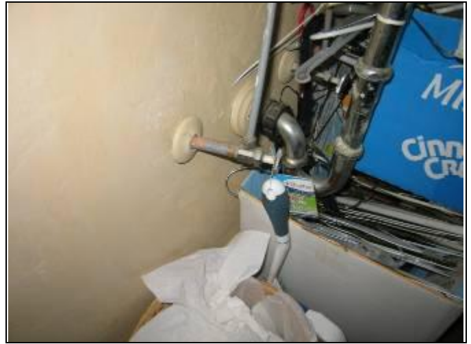
50. Polybutylene water distribution piping at toilet lavatory Building 113
