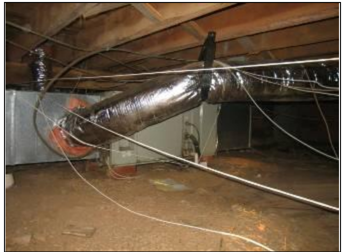
40. One of two heat pump Air Handler units in Building 115 crawlspace
