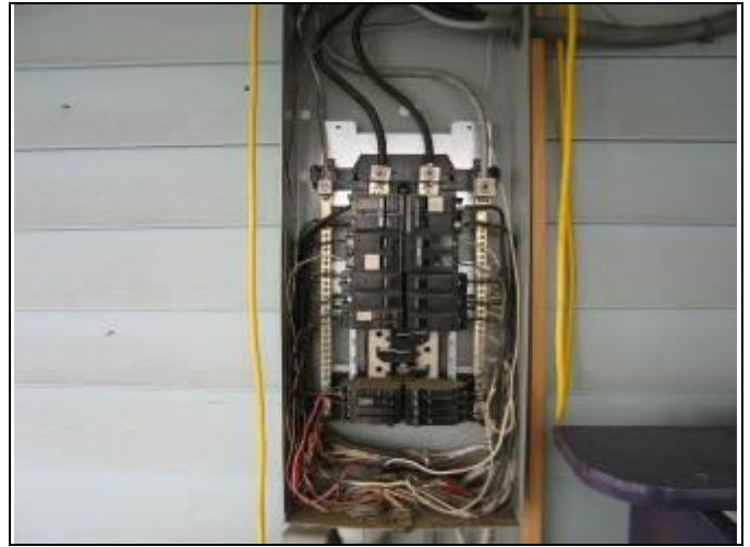
44. Distribution panel at Building 113 – breaker at upper left is off but feeds unsecured/unused cable
