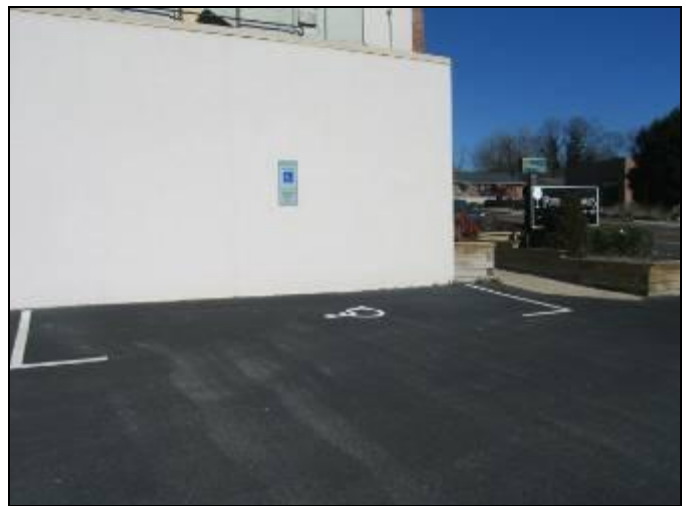
16. ADA designated at Building 115 not Van Accessible sized and inaccessible route (step up)
