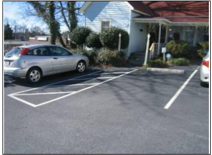
14. Building 113 parking – no ADA designated Van Accessible
