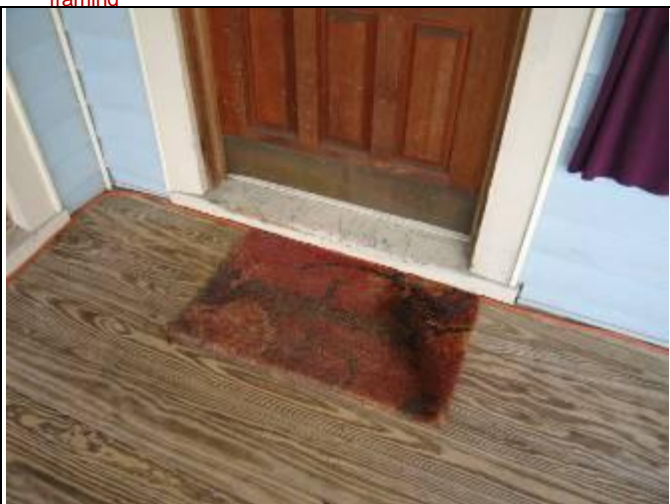
71. ADA accessibility view 1: Front entry threshold at Building 113 in excess of 3/4 inch and generally not negotiable by unassisted wheelchair - additional short ramp needed
