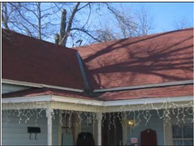
33. Building 113 relatively new asphalt shingle roof with metal valley flashing and no gutters installed
