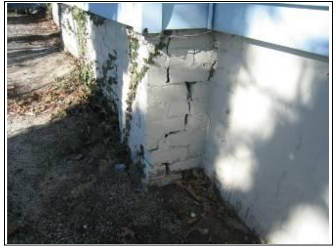
62. Structural view 9: Degradation of 111 year old brick pier at building 113 to be expected
