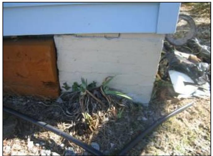
64. Structural view 11: Left rear corner pier rotated – see prior caption
