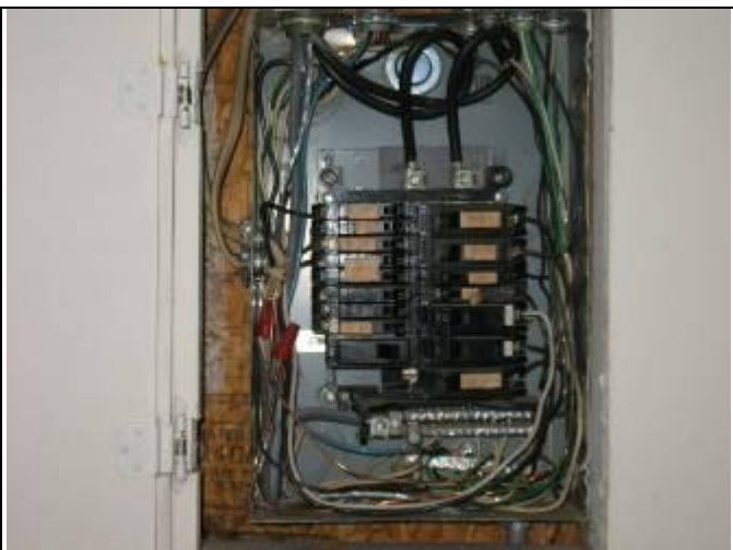
45. Older service panel at unit C Building 115 – no aluminum distribution wiring noted in any panel
