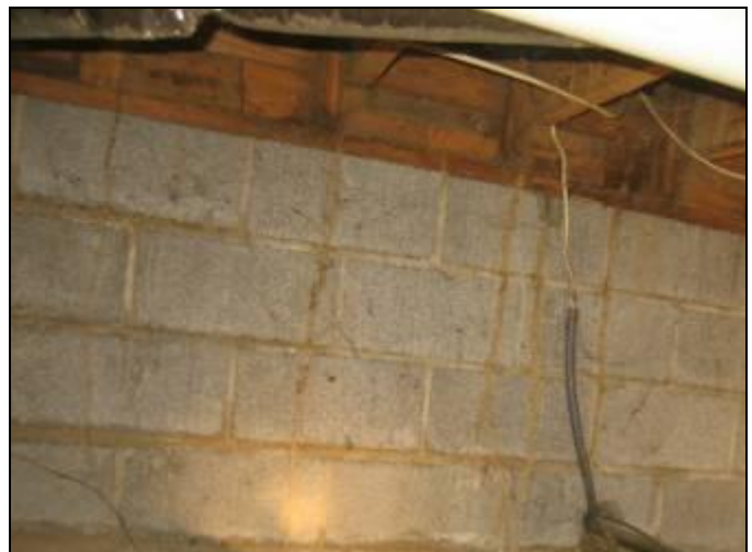
58. Structural view 6: Prior termite activity (tubes) in the 115 Building crawlspace – no cracking noted in foundation walls
