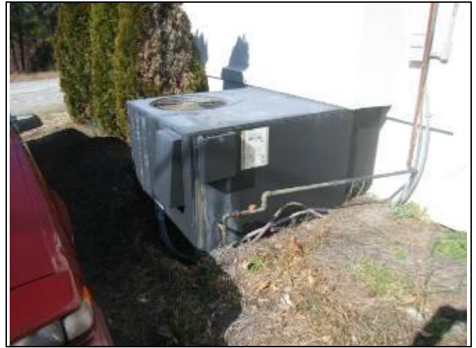
38. Gas pack HVAC unit for tenant space D – leaking natural gas at area of shut off valve
