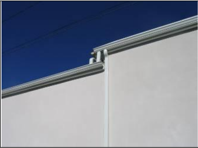
31. Three gutters point of discharge at Building 115 south elevation
