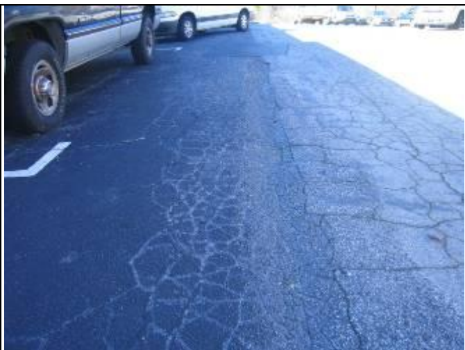
21. Deteriorated asphalt at Building 115 north parking lane
