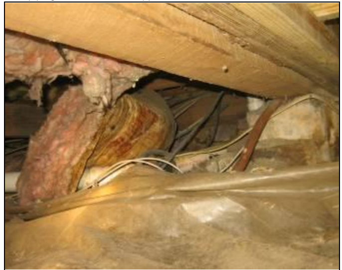
70. Structural view 17: Building 113: Distribution wiring improperly installed, displaced or improperly installed insulation, more debris, etc - safety concern
