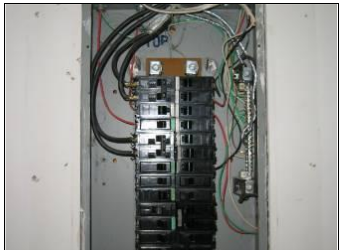
46. Newer breaker panel in unit B - Building 115 has loose breaker/buss assembly
