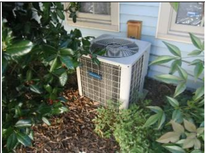
41. Split system air conditioner condensing unit at Building 113 – mfg 1995 by Comfortmaker
