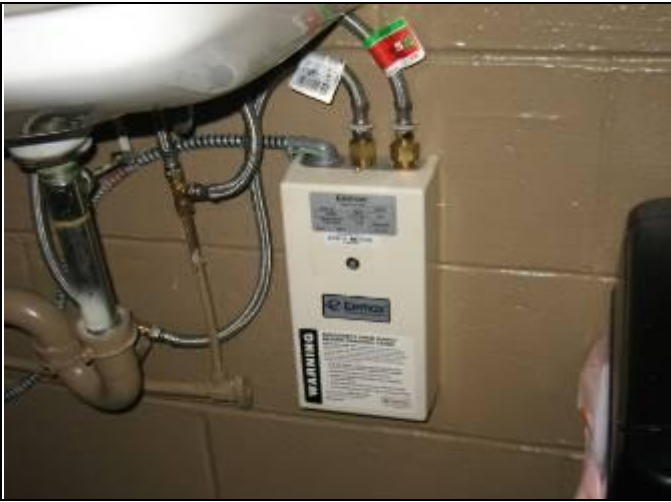
49. Tankless “on-demand” water heater for unit A - Building 115 public toilets
