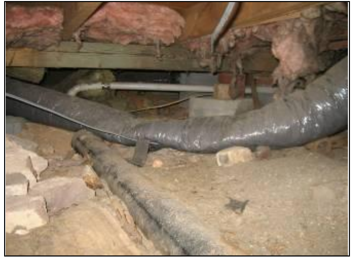
68. Structural view 15: Building 113 Crawl space: Displaced insulation, crushed HVAC supply duct, debris, PVC and Cast Iron waste piping, additional floor supports of stacked materials
