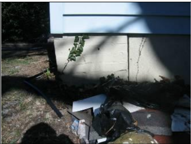
63. Structural view 10: Left rear corner pier rotated outward likely due to moist footings
