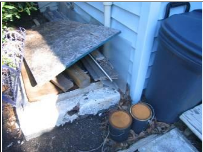
65. Structural view 12: Debris collection prevents examination of exterior wall and encourages intrusion by insects and other undesirables including water.
