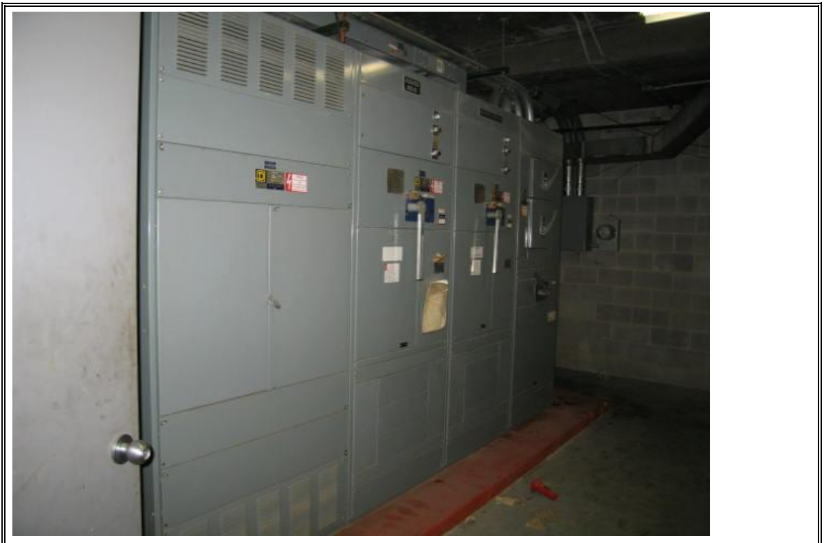
Photograph Number 8: Subject building main switchgear
