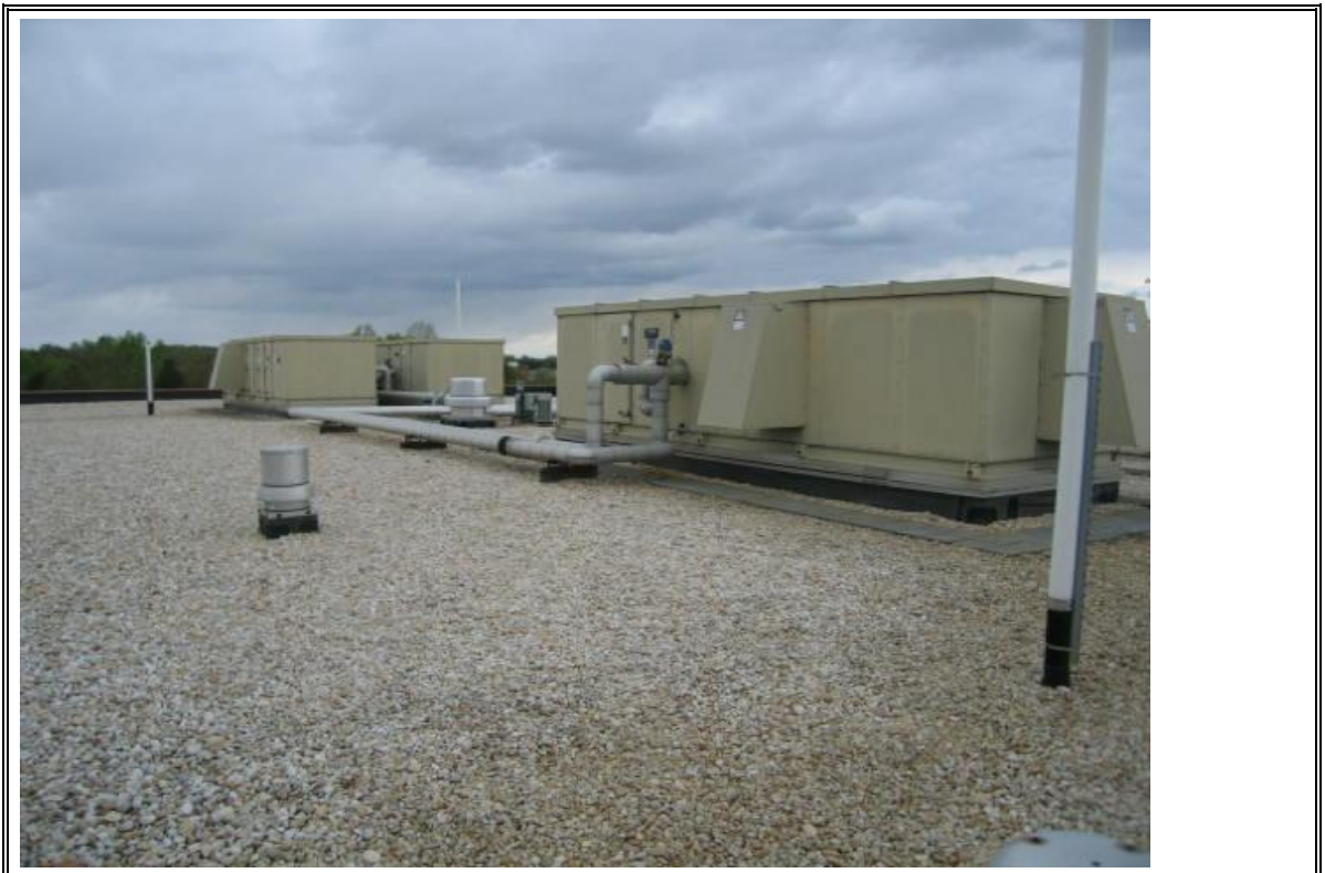
Photograph Number 4: Rooftop view of HVAC systems
