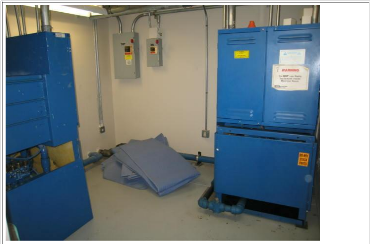
Photograph Number 9: View of dual hydraulic elevator pump/control area
