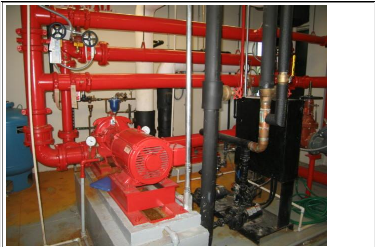
Photograph Number 10: View of typical wet pipe sprinkler system with electric fire pump
