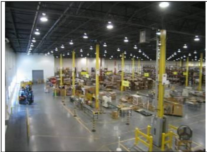
21. Manufacturing area - note typical switchgear
