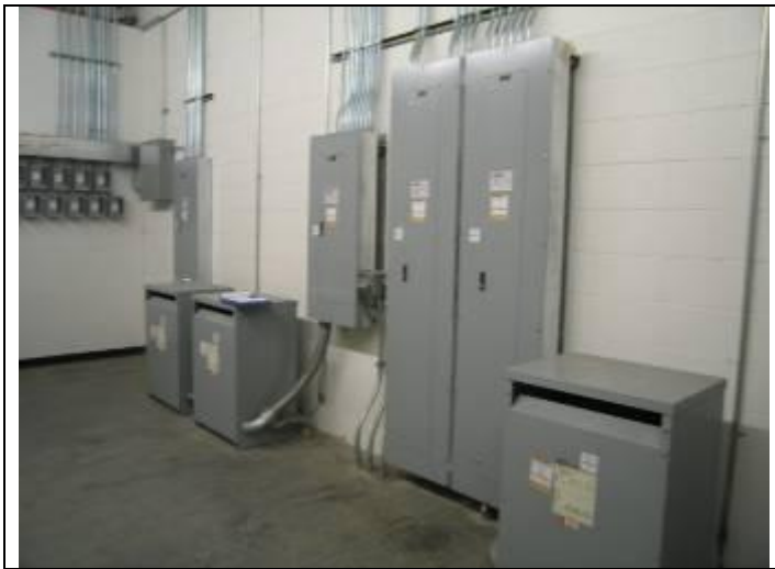
27. 2000 ampere 480 V switchgear (one of two mains)
