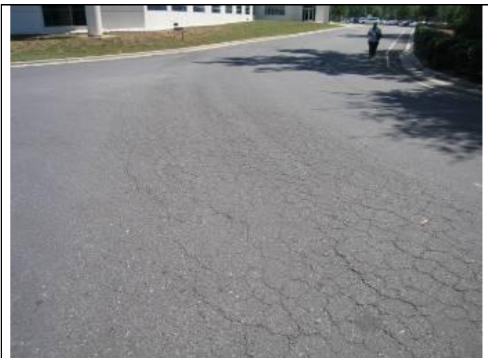
3. Alligatored asphalt at main driveway entry -
