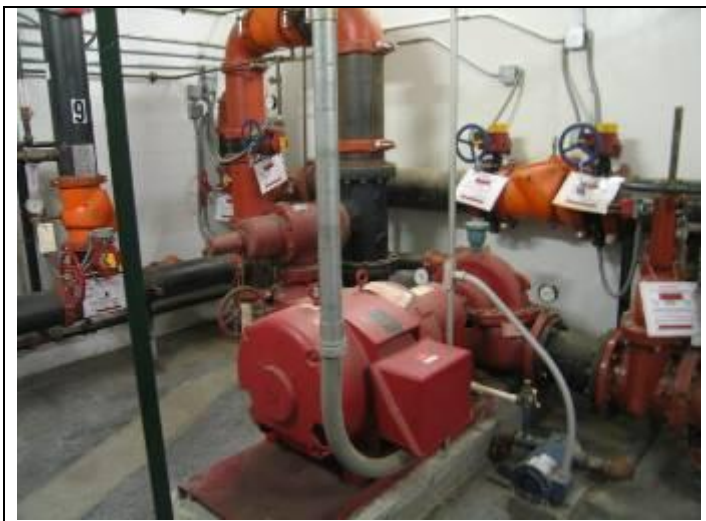
29. 150 hp fire pump and ancillary equipment
