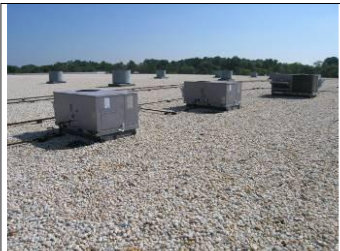
39. Rooftop northeast view –RTUs
