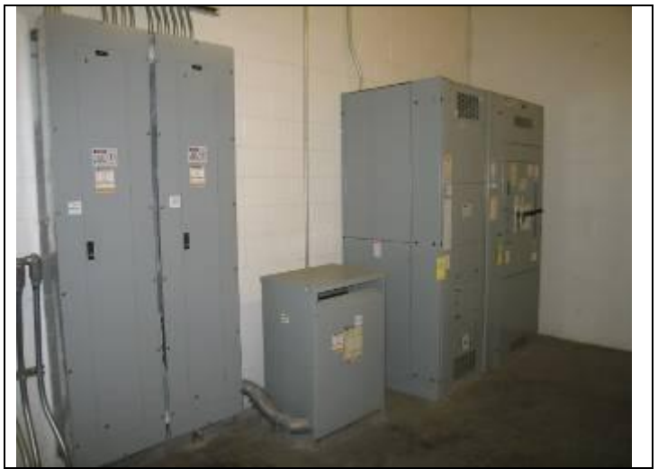
26. 2000 ampere 480 V switchgear (one of two mains)
