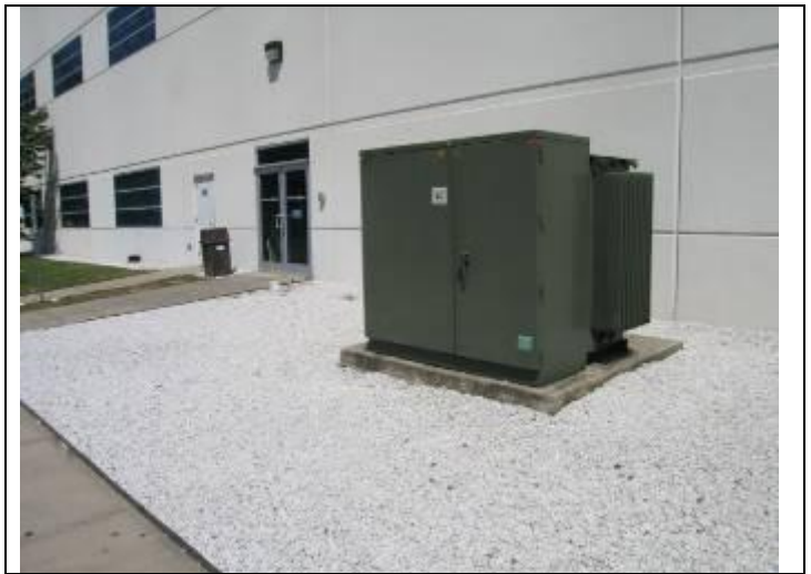
28. Pad mounted utility transformer 750 kVA 480 V
