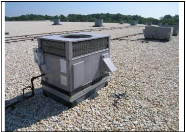
38. Rooftop package unit (natural gas fired)
