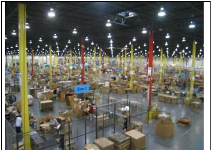
22. Sprinkler risers w/hose on red columns
