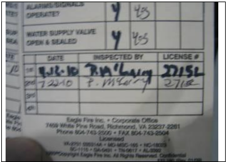
32. Current sprinkler riser inspection tag
