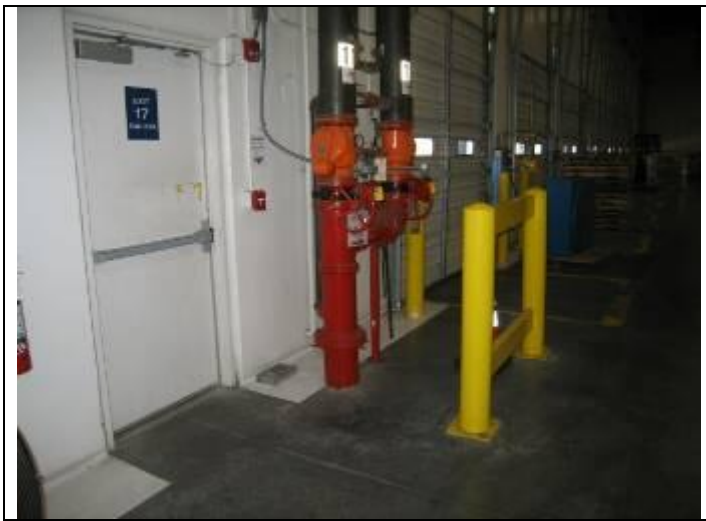
31. Sprinkler riser (one of two similar)
