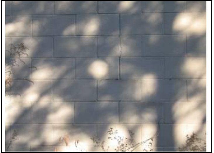
22. Through-block and stair-step cracking at south elevation
