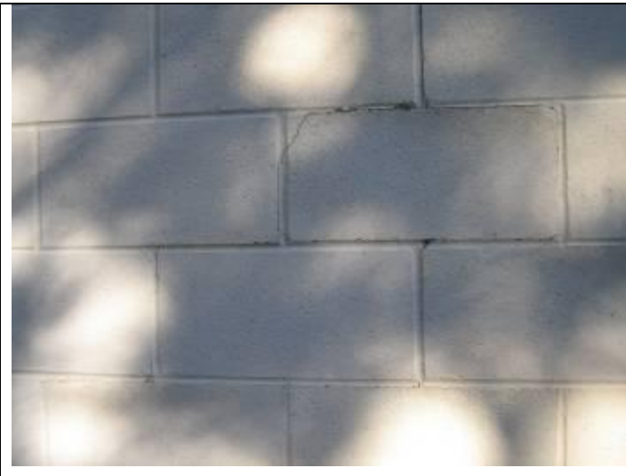
23. Through-block and stair-step cracking at south elevation
