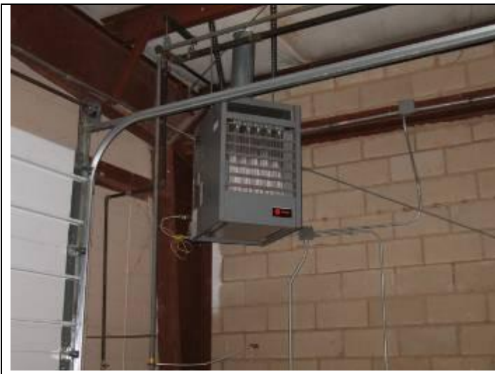
37. Natural gas fired space heater (gas supply design capacity is for two heaters per construction drawings)
