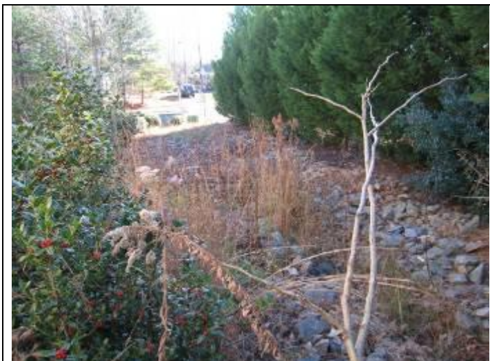
17. Rip-rap lined drainage ditch at south parcel border and parallel to south building elevation
