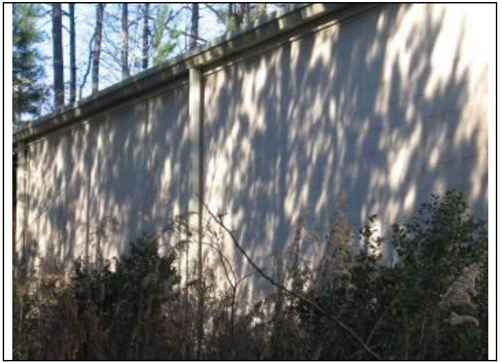
20. Area of wall separation/settlement
