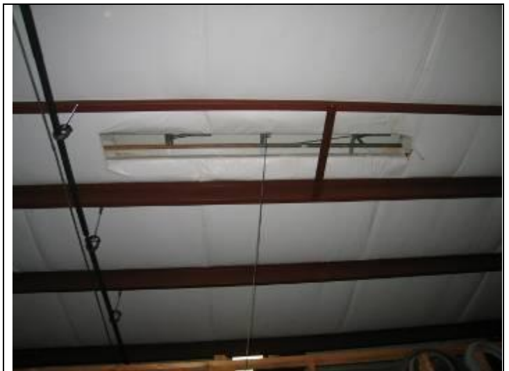
38. ceiling located manual ventilation (one of two)
