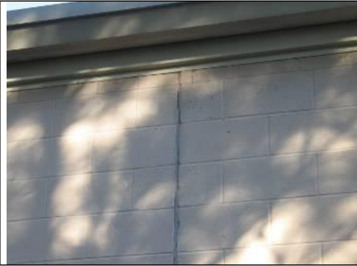
21. Separation of south elevation expansion joint
