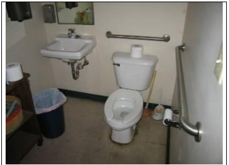
40. ADA toilet for warehouse staff
