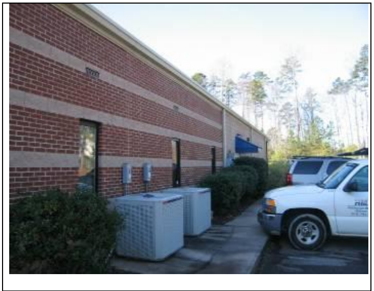
2. Right side (north) elevation – twin split heat pumps and utilities
