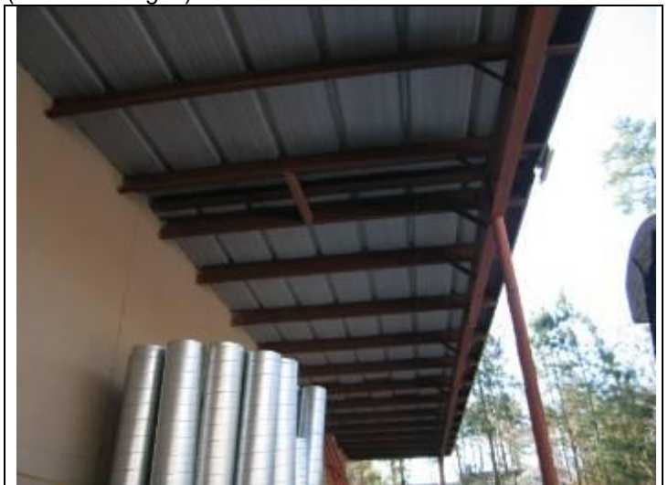
16. Canopy framing in good condition – some loose metal trim at upper right
