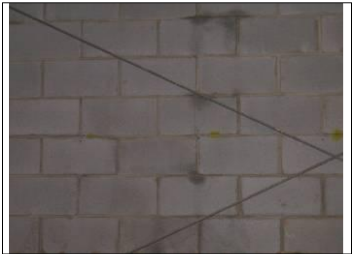
26. South elevation wall interior view with cracking through block at upper center and continuing in stair-step
