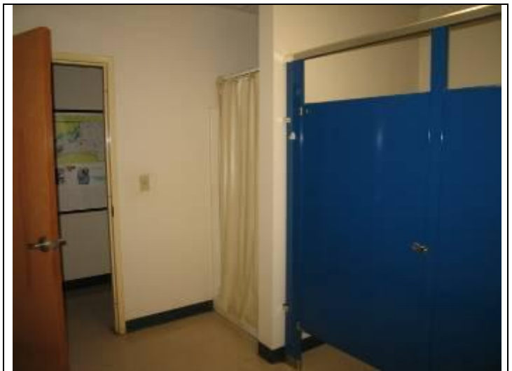
32. ADA toilet entry at
