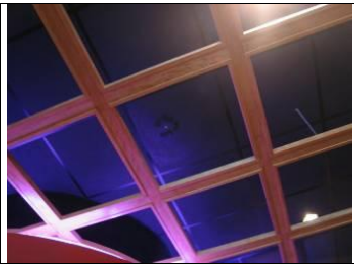
25. One of two reported active roof leaks at HoBoy Steakhouse
