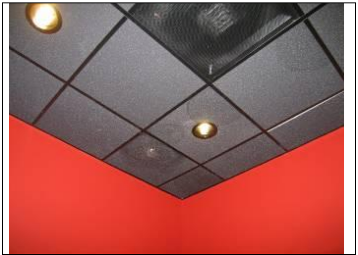
26. One of two reported active roof leaks at HoBoy Steakhouse
