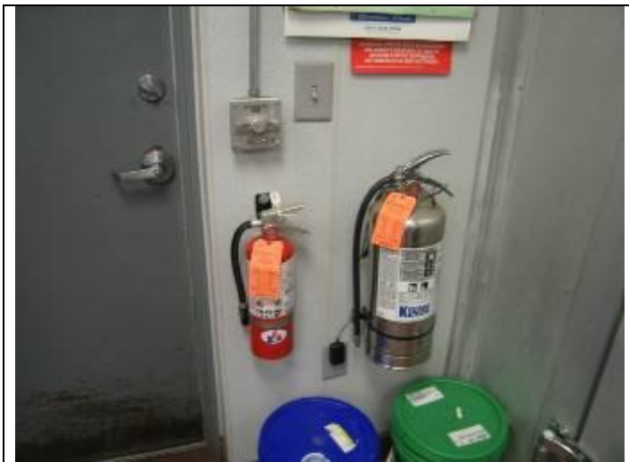
39. Exhaust hood extinguisher pull station typical
