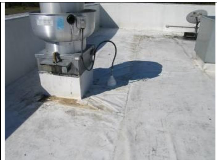
45. Building 5916 possible grease overflow above unit 110
