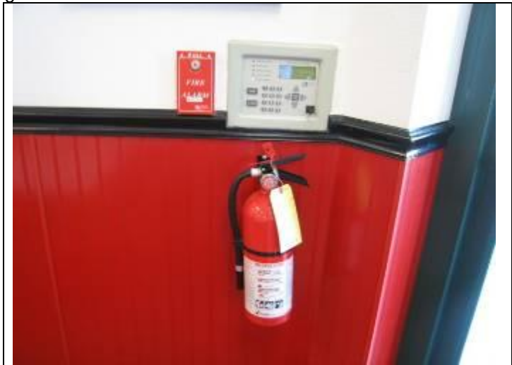
34. Building 5920 fire controller in unit 170 – current ext. tag
