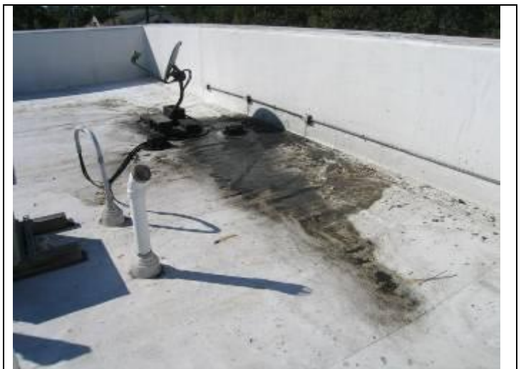
46. Building 5916 grease accumulation above unit 110
