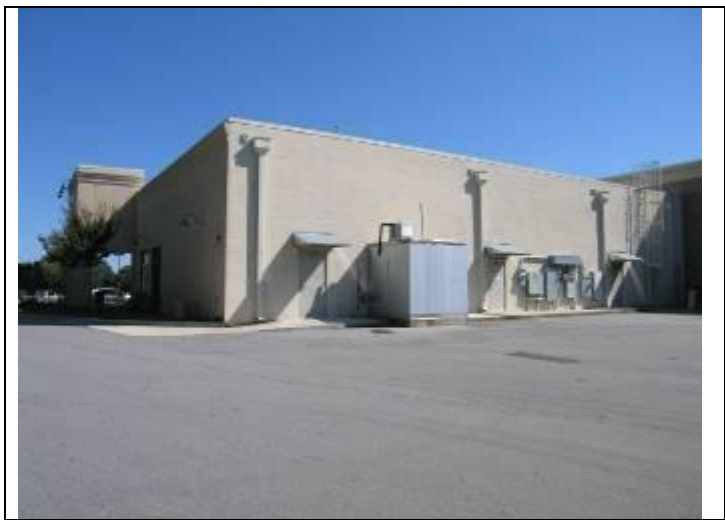
16. Bldg 5920 units 140,160,170 – Sprinkler riser inaccessible
