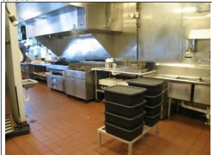
35. Building 5916 unit 110 MB's Grille kitchen view
