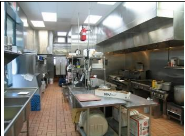
23. HoBoy Japanese Steakhouse kitchen in good condition
