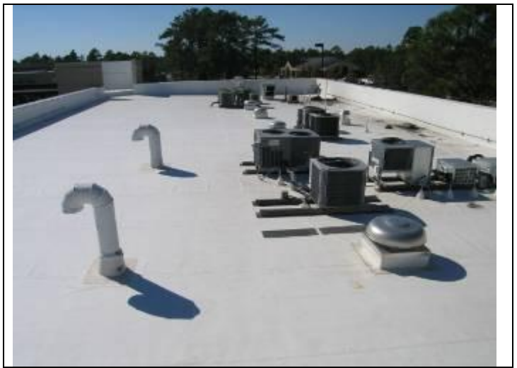
44. Building 5916 above units 110 (far), 120, 130 & 150
