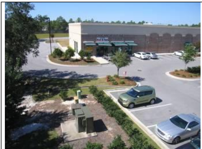
11. Bldg. 5920 Longer Nails w/o close ADA prkg - site xfmr typical
